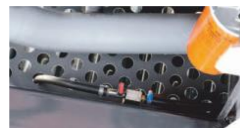
Fuel tank water drainage cock
