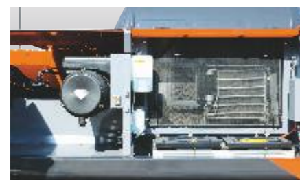
Utility space and radiators
