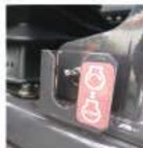
Emergency engine stop switch
